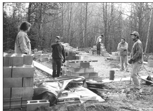
Jim, Rick, Randy & Mike worked hard one Saturday, laying the block for the new cabin foundation.
