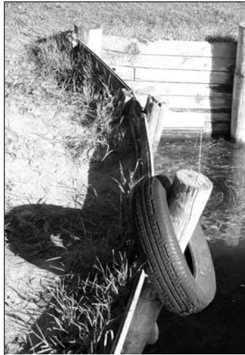
The harbor walls have been caving more each year. Anchor cables have slipped, poles are weakening and the original design and installation has not withstood the pressure.
